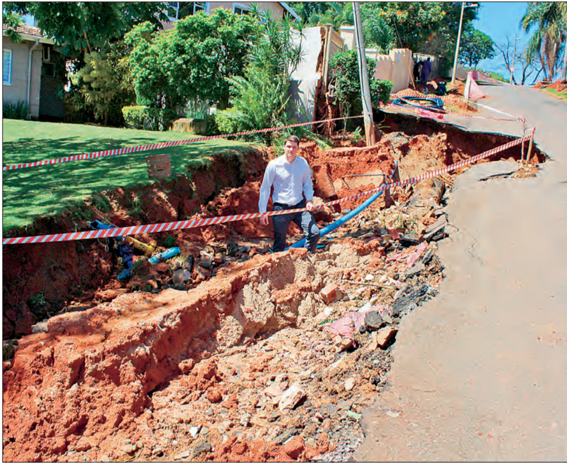
A large section of Melrose Avenue has been severely undermined by several burst pipes. Durban North ward councillor, Shaun Ryley, said residents were irate over the damage done to the road and their properties.
